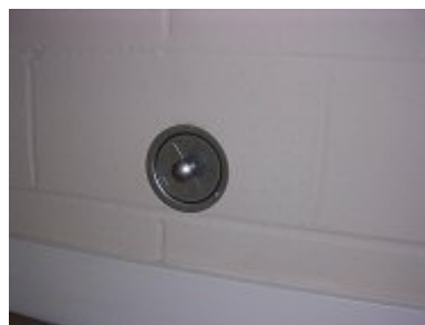
Air vent closed
